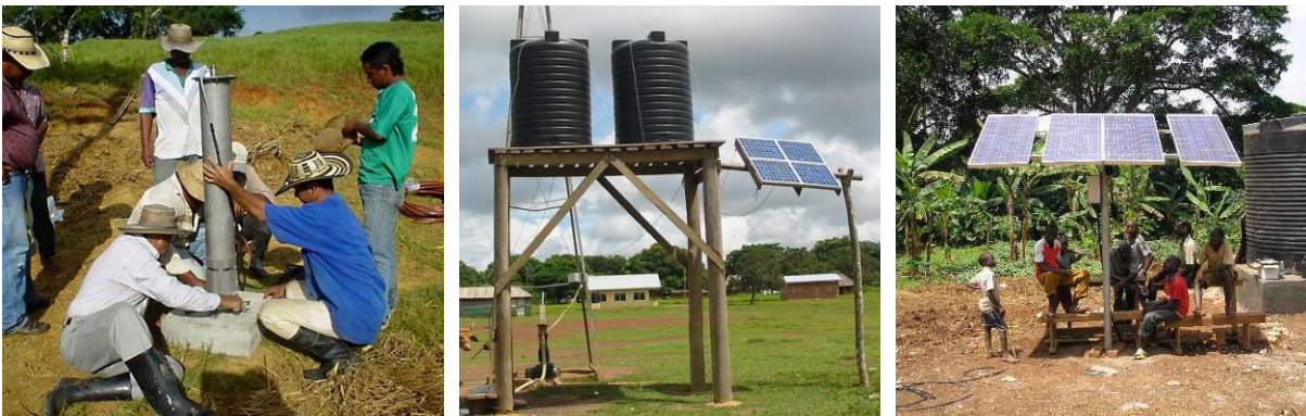
Simple installations provide stable, efficient water supply
