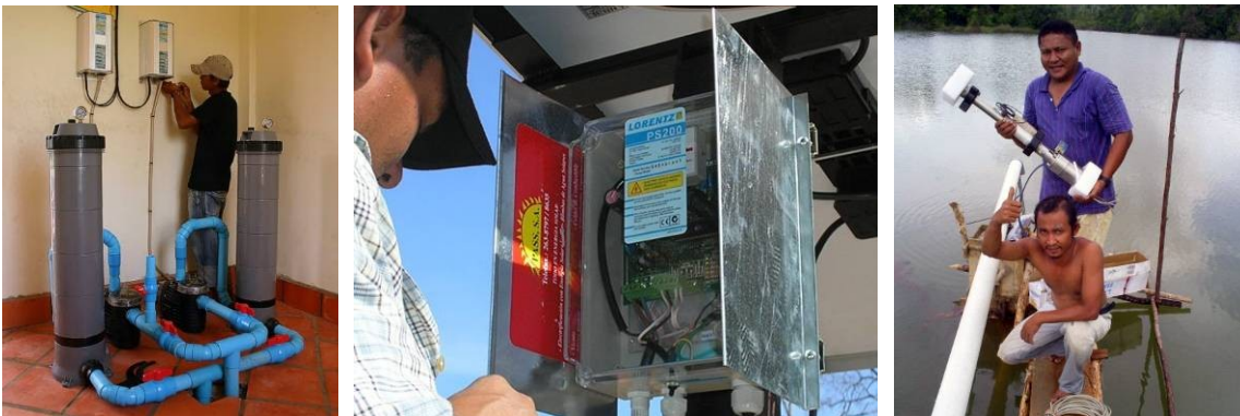
LORENTZ systems are installed in more than 100 countries all over the globe
