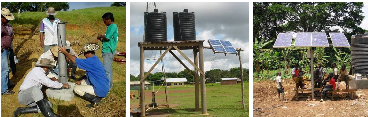
Simple installations provide stable, efficient water supply
